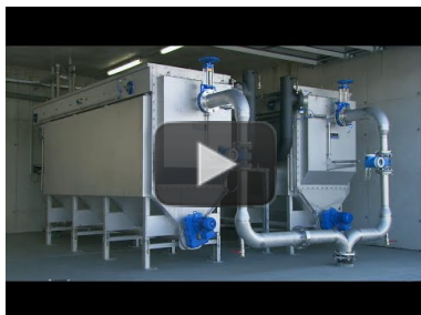
Video: HUBER Solution ThermWin® for Heat Recovery from Sewers
