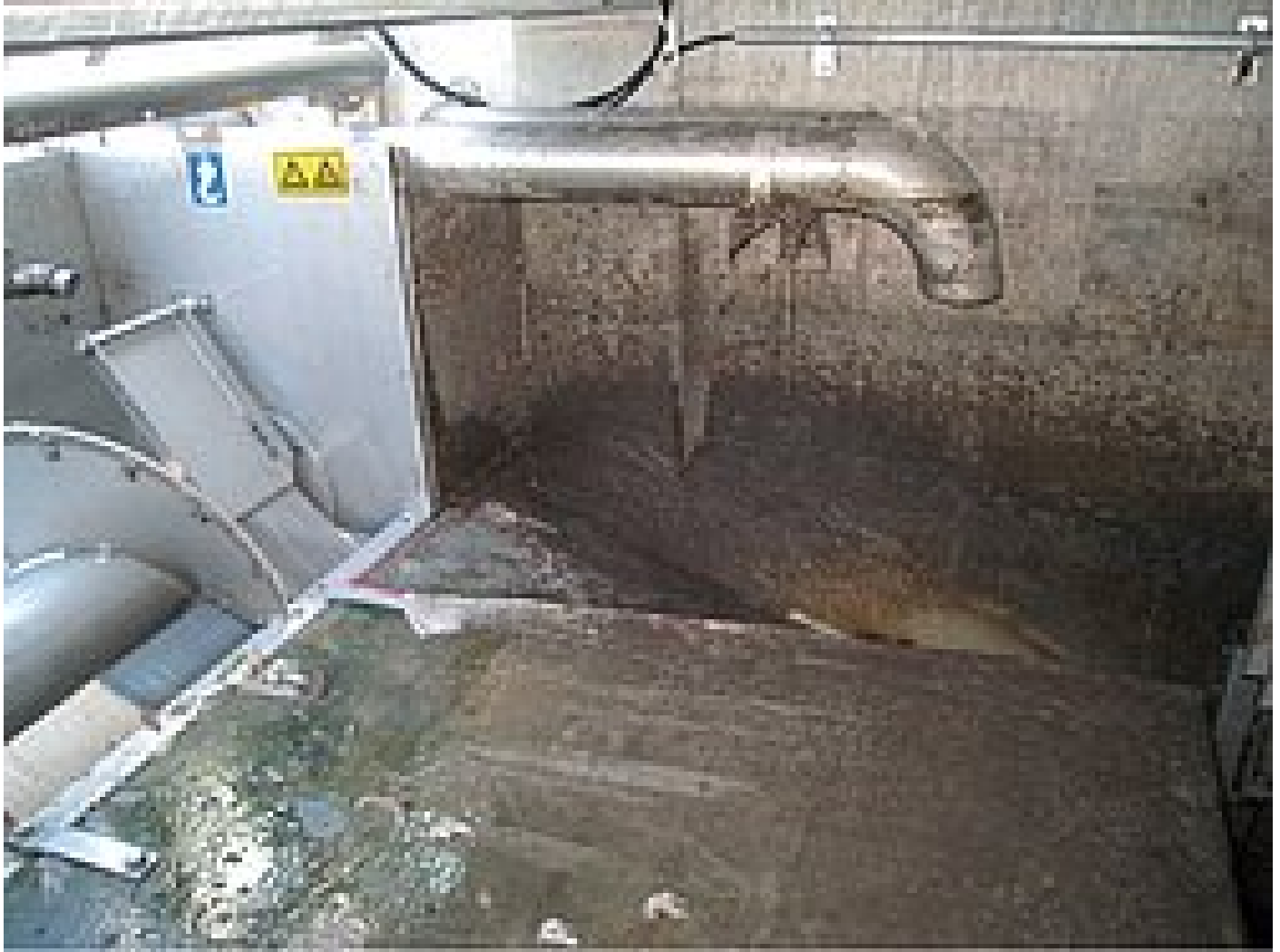
Screening launder channel built into the berm, washing system at the left, discharge line on top
