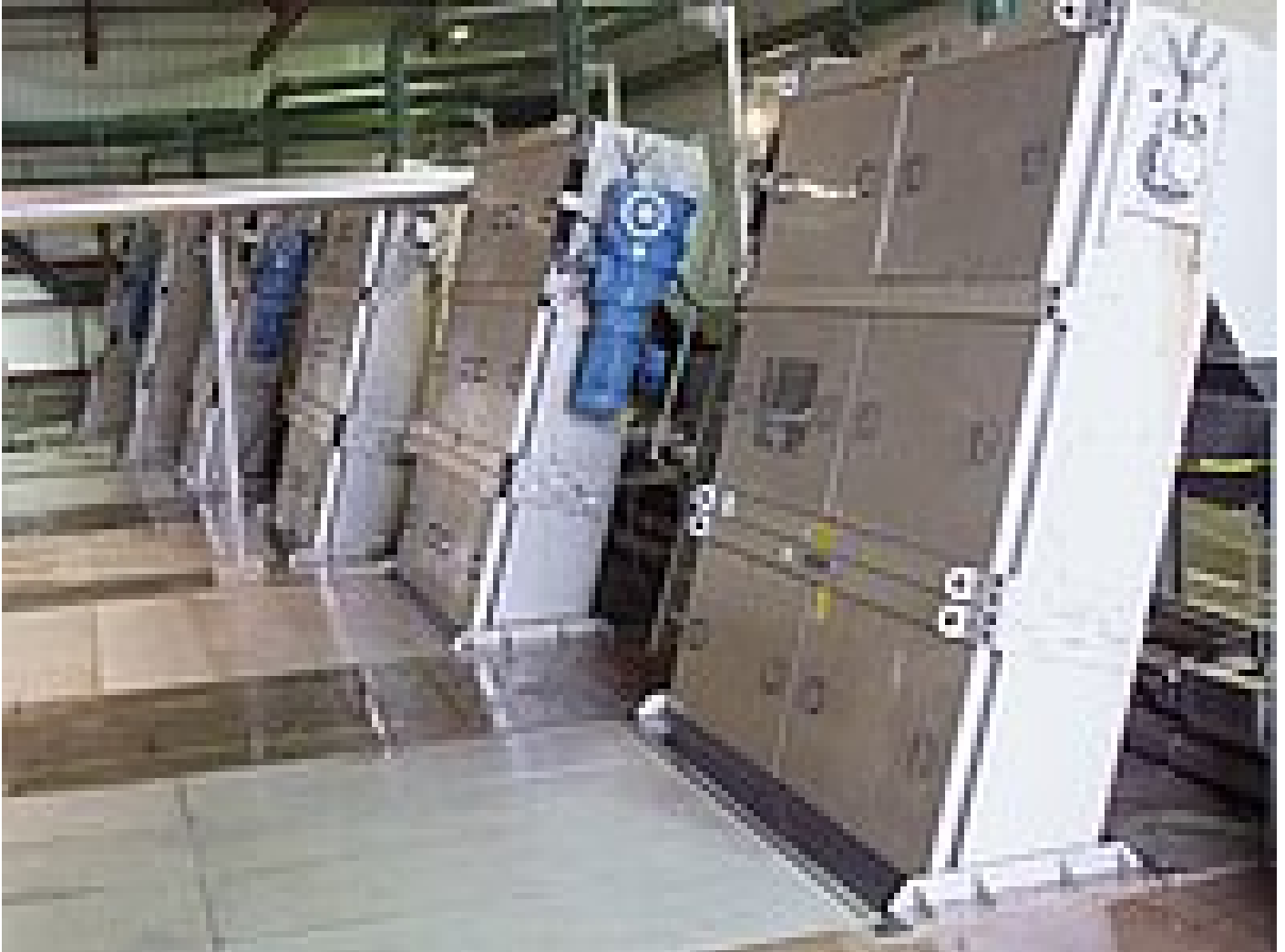
Tops of the seven RakeMax® multi-rake bar screens
