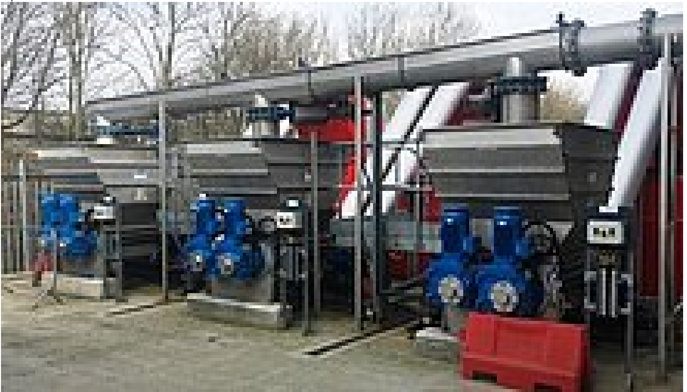
Coarse screens low level launder and WAP@ SL 12v wash presses
